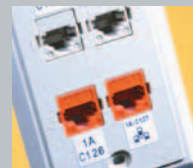
Patch Panel & Faceplates
