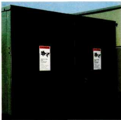
"Mr. Ouch" Transformer Markings effectively warn children to stay away from pad mounted transformers.
